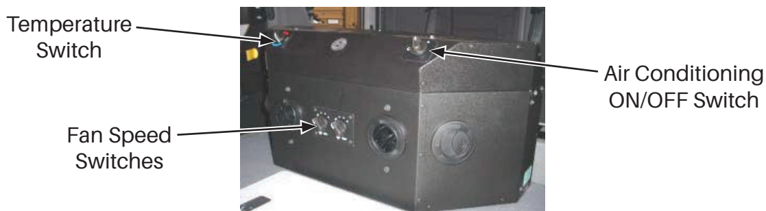
Figure 3-53. Tunnel Mounted HVAC System
