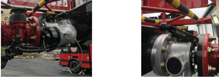
Figure 4-14. Aerial Standpipe Connection
